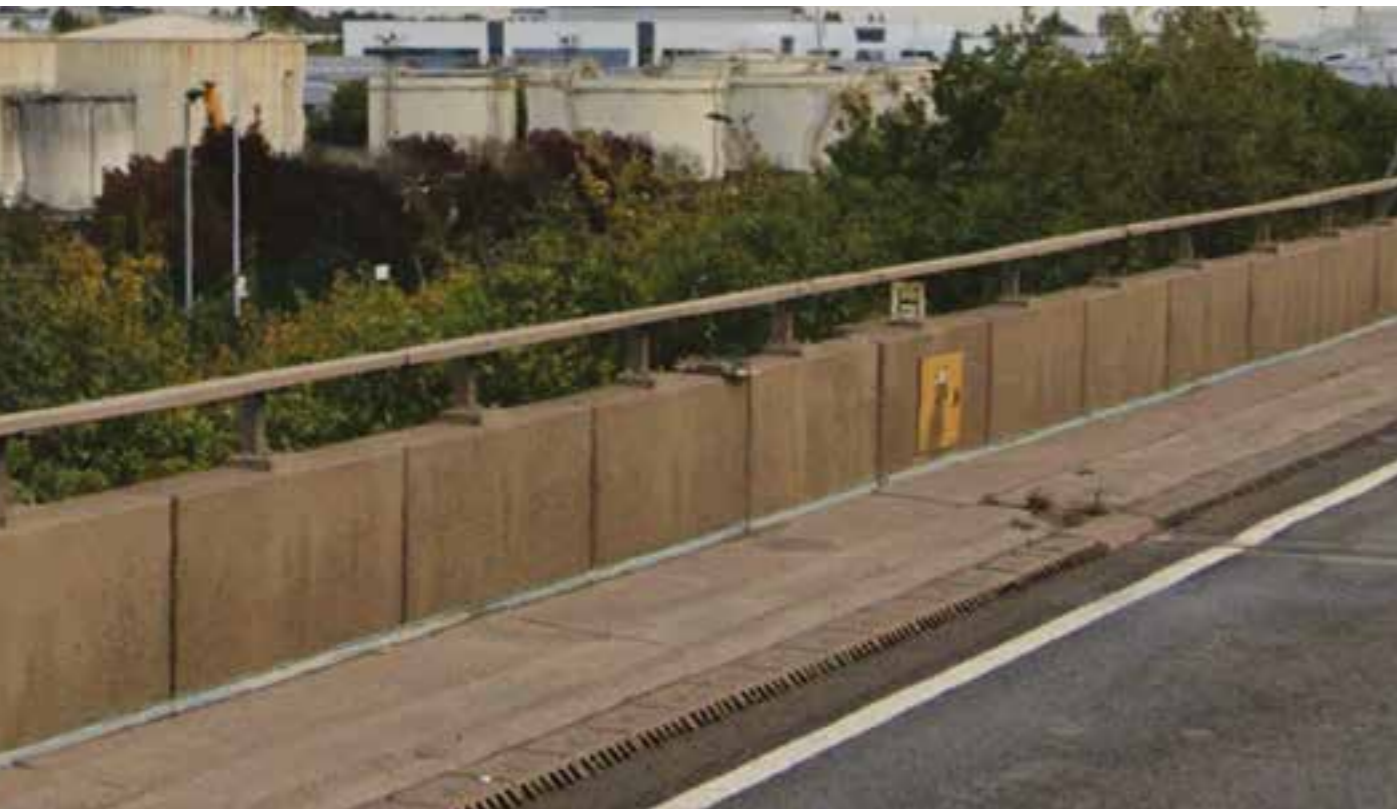
Figure 4 1.2 metre kerbed area between the edge of the carriageway and the parapet © Google
