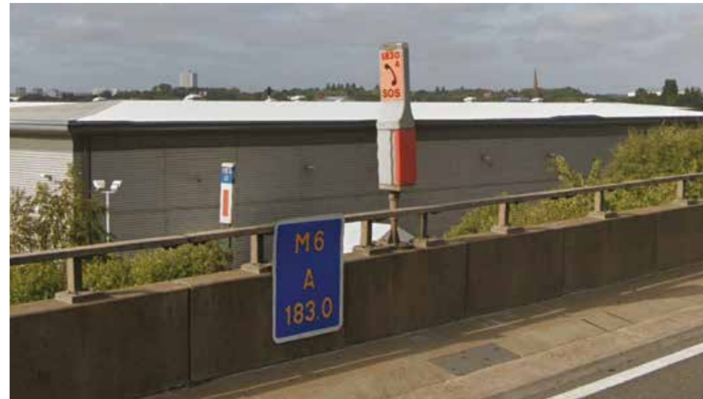
Figure 3 Parapet mounted emergency roadside telephone on Bromford Viaduct © Google
