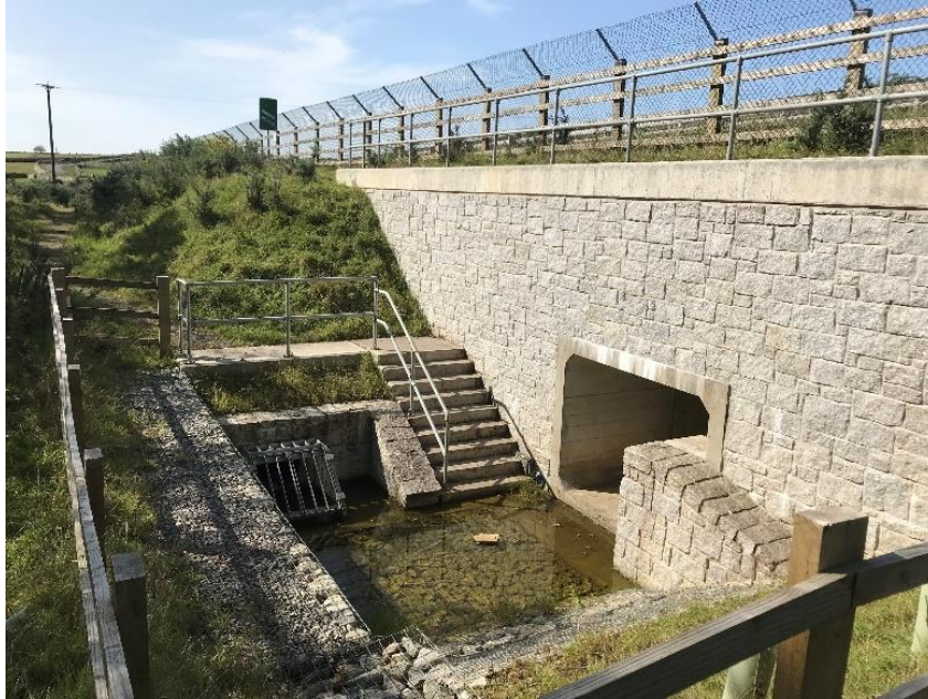
Figure 21 Otter fencing and mammal ledge within culvert at Pounds Conce
